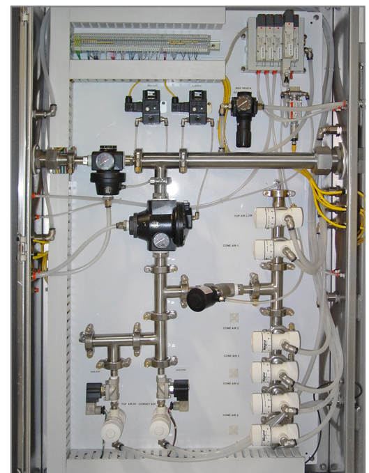
Compressed air control panel
