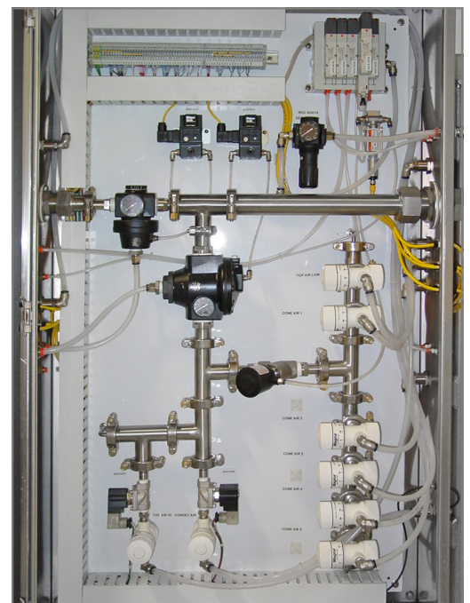
Compressed air control panel
